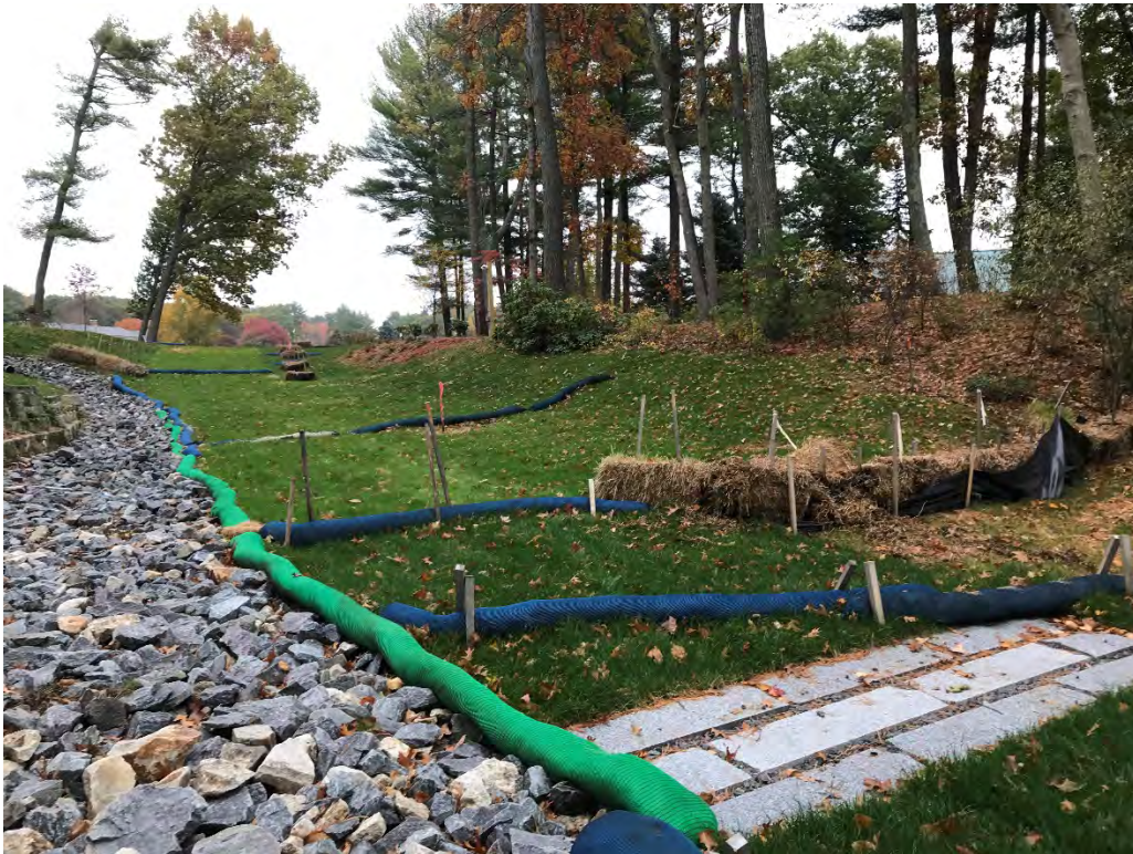
Fig 8: Slope above the manhole at Gundalow Landing/east side of the bay. Viewing east. (10-21-20)
