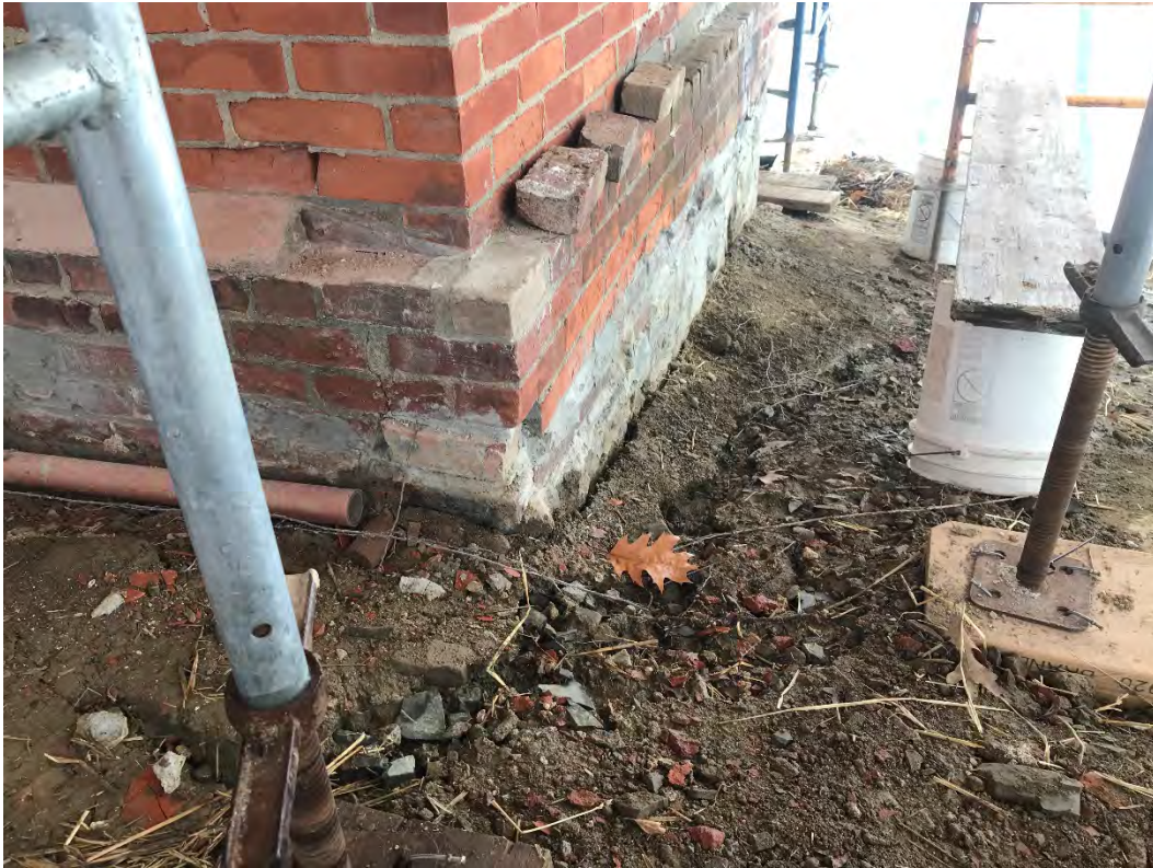
Fig 5: Rill observed on the southwest corner of the cable house at the Eversource property/west side of the bay. Viewing east. (10-17-20)
