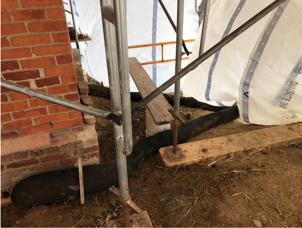
Fig 7: Repaired rill and silt socks off the southern side of the cable house at the Eversource property/west side of the bay. Viewing southeast. (10-19-20)
