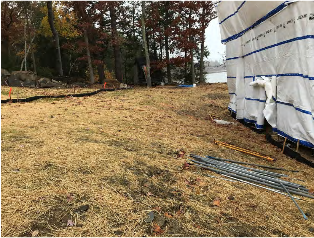
Fig 1: Slope above the cable house at the Eversource property/west side of the bay. Viewing north. (10-21-20)
