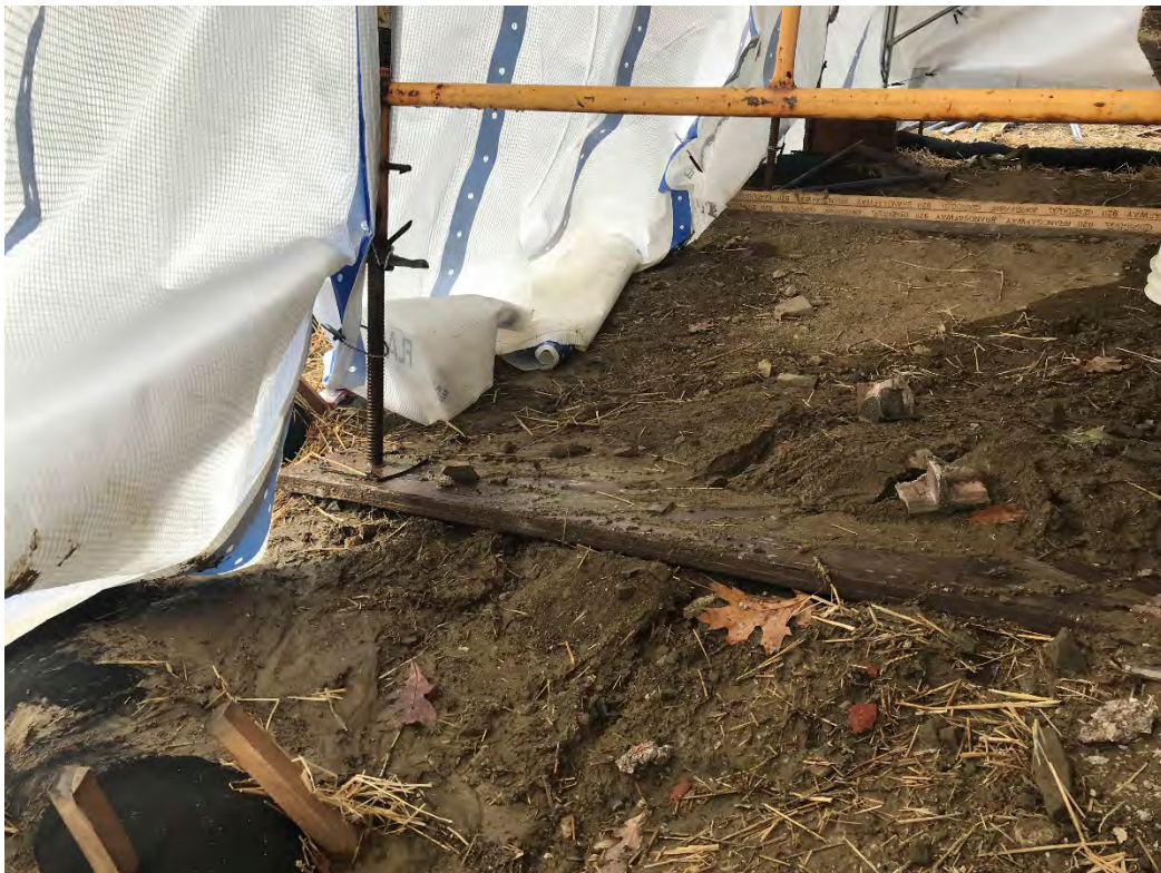
Fig 6: Rills observed off the southeast corner of the cable house at the Eversource property/west side of the bay. Viewing southwest. (10-17-20)
