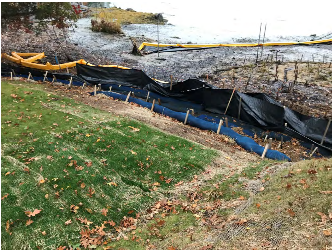
Fig 10: Toe of the slope at Gundalow Landing/east side of the bay. Viewing south. (10-21-20)
