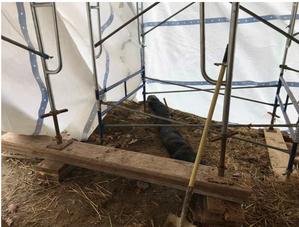
Fig 4: Repaired rill and silt sock off the northeast corner of the cable house at the Eversource property/west side of the bay. Viewing east. (10-19-20)
